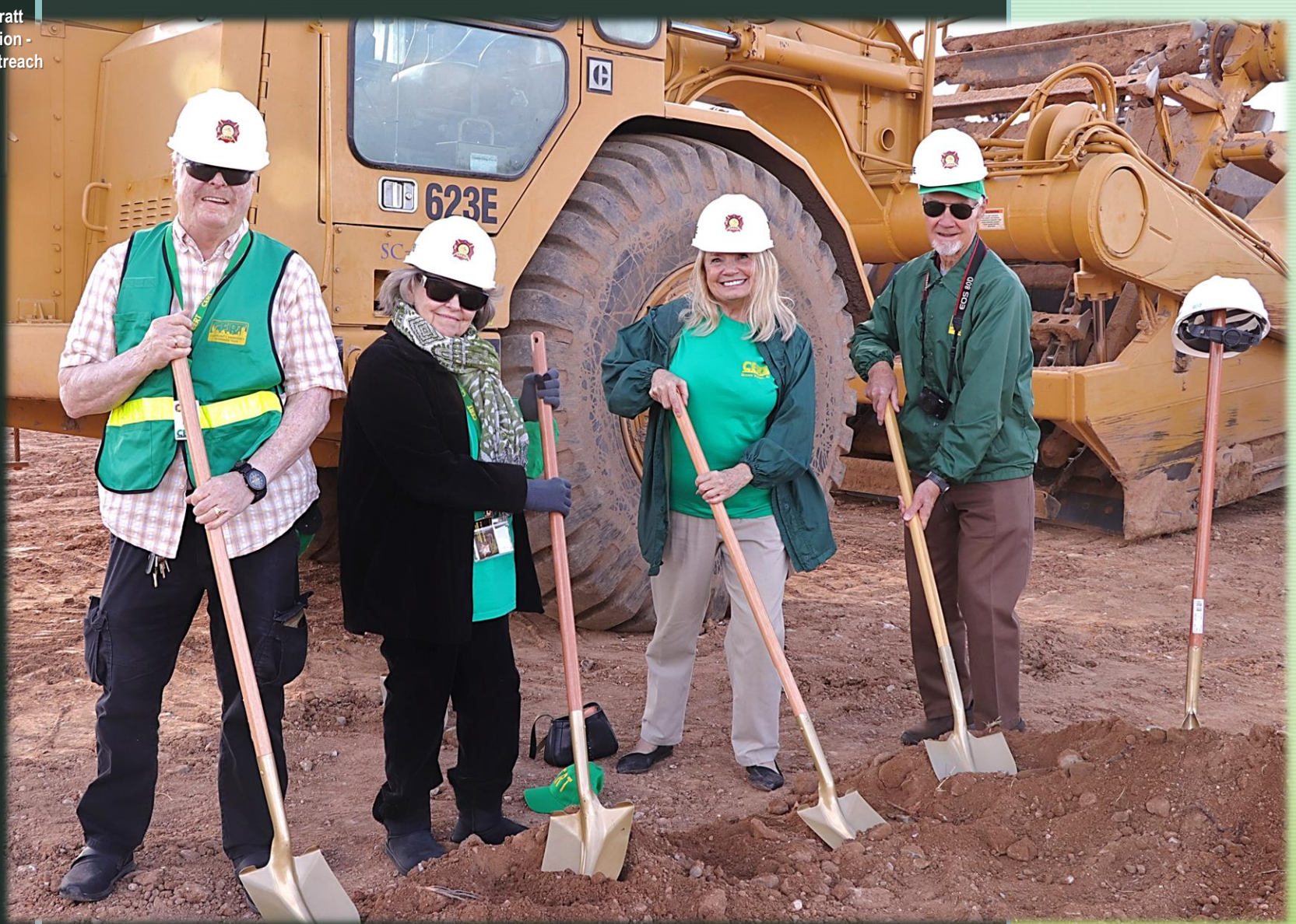
CERT members break ground for new GVFD Station 152, January 5, 2023. From left to right: Paul Fitch, Carol Petty, Judy Schmidt, John McGee. Scheduled completion in late 2023.
